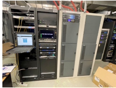
Tx Chain and Power Amp
